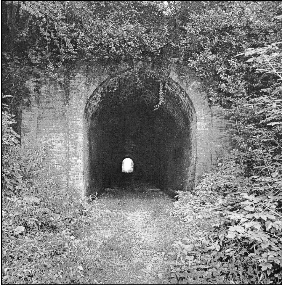
Railway Tunnel under Melbourne road, Newbold – Southern Entrance Photograph c.1971 – After rails were removed
