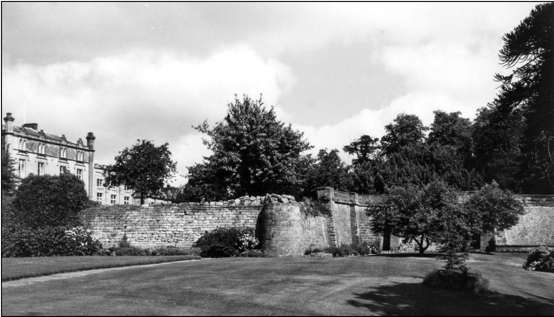
4m high retaining wall viewed from the Winter Garden area in 1984, with the Hall in the background.
