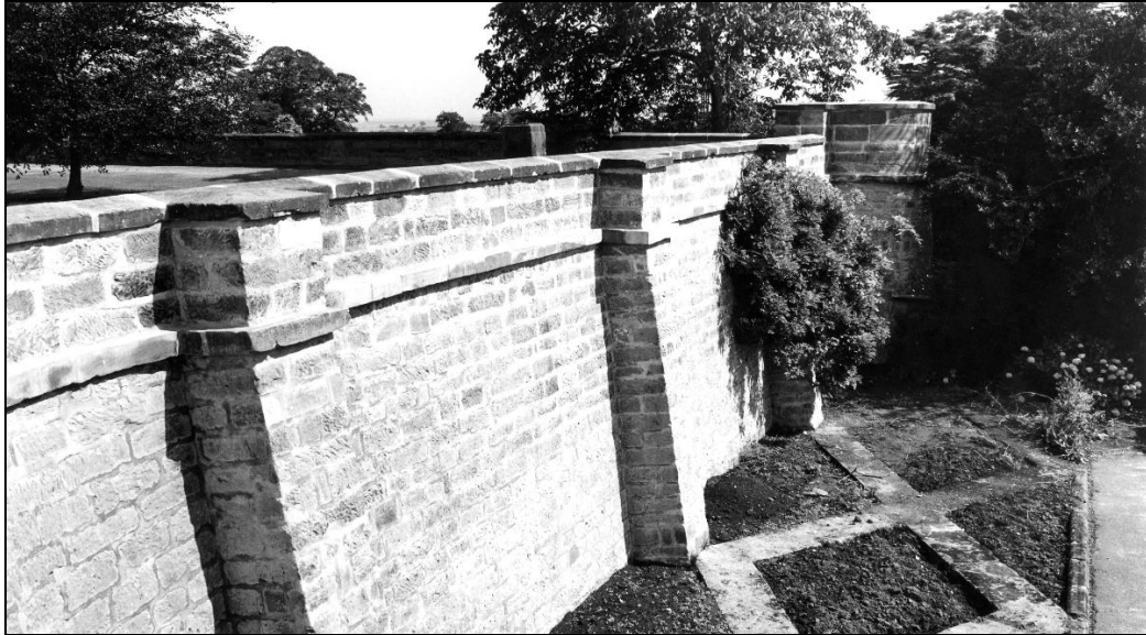
Eastern end of the 4m high retaining wall with a viewing "Pulpit" at the end. This is shown on Wordsworth's plan at the north east corner. This photograph was taken after repairs to the wall were carried out in 1986.
