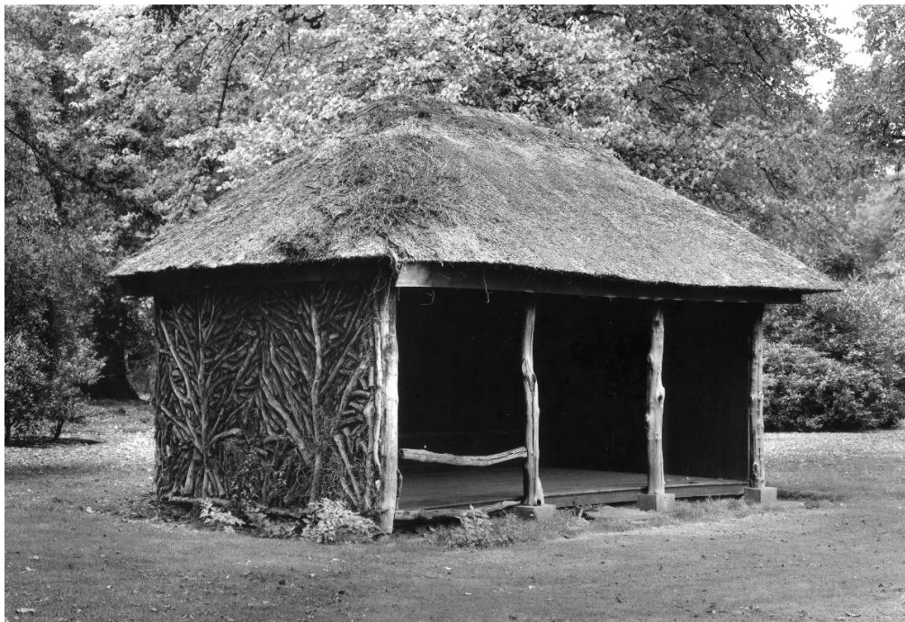
The summerhouse in poor condition in 1994. This was perhaps a copy of the previous summerhouse shown in the earlier John Mathews map. The date it was built is not known .
